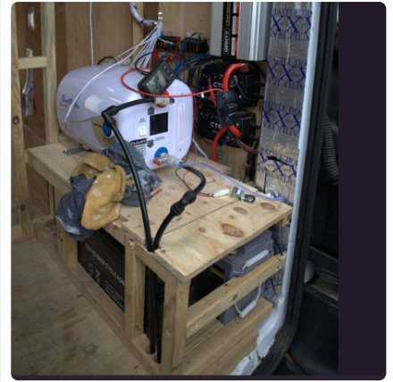
Testing mode hot water tank.
