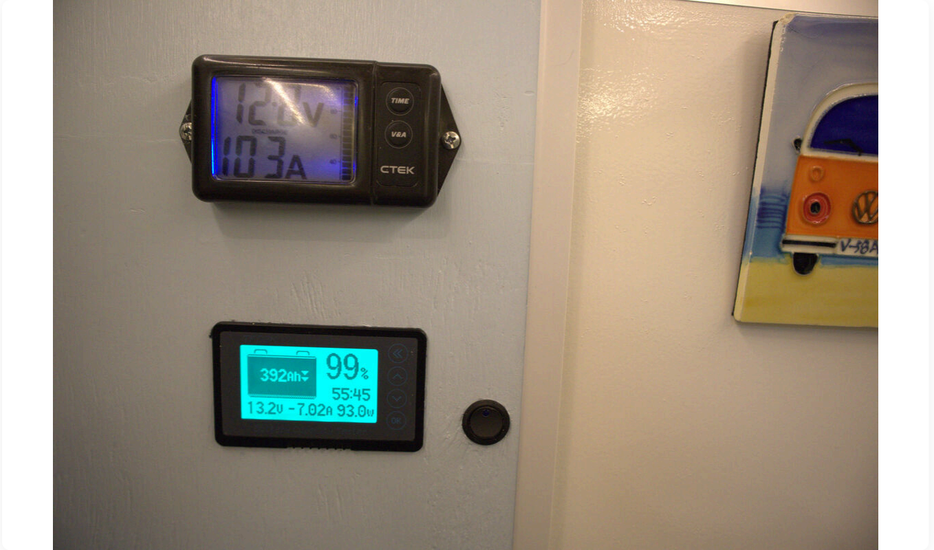
Dual solar readout displays — monitoring the full system
